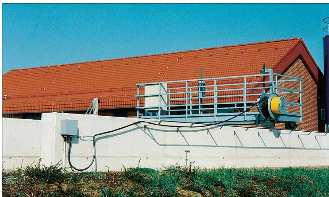
Main spring cable power feed for a skimmer in a water treatment facility.
